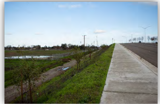
Figure 3 - Capital improvement projects such as roadways must include post-construction design measures and be appropriately sized.
